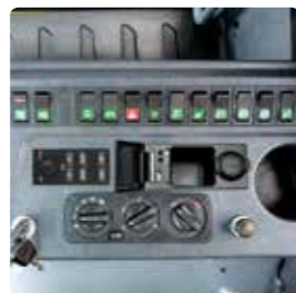
Centralized Instrument Switch Panel
